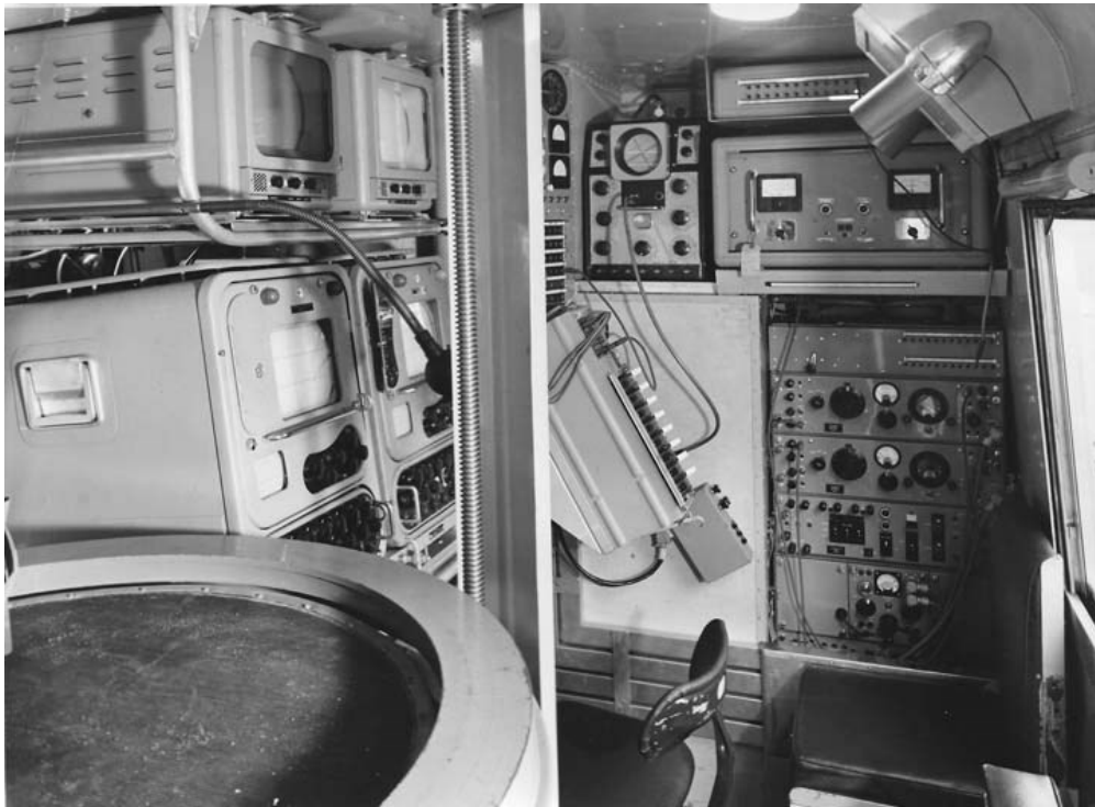
Internal arrangement of equipment. Camera control monitors and radio check monitors on the left; sound communication equipment on the right. Left foreground: camera lift,; centre top: aerial bearing dial
