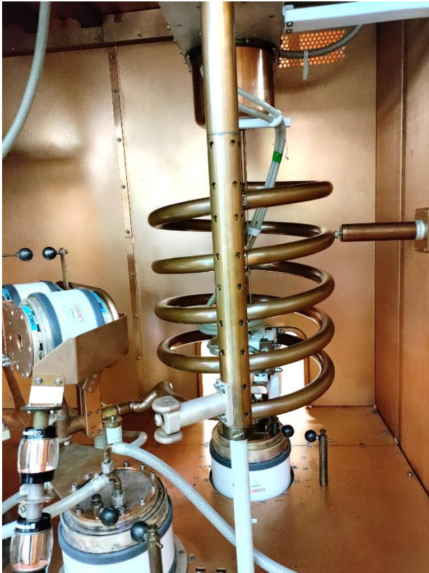
Figure 8. Close-up of L308, coupling capacitors and M13 motorised coil short
