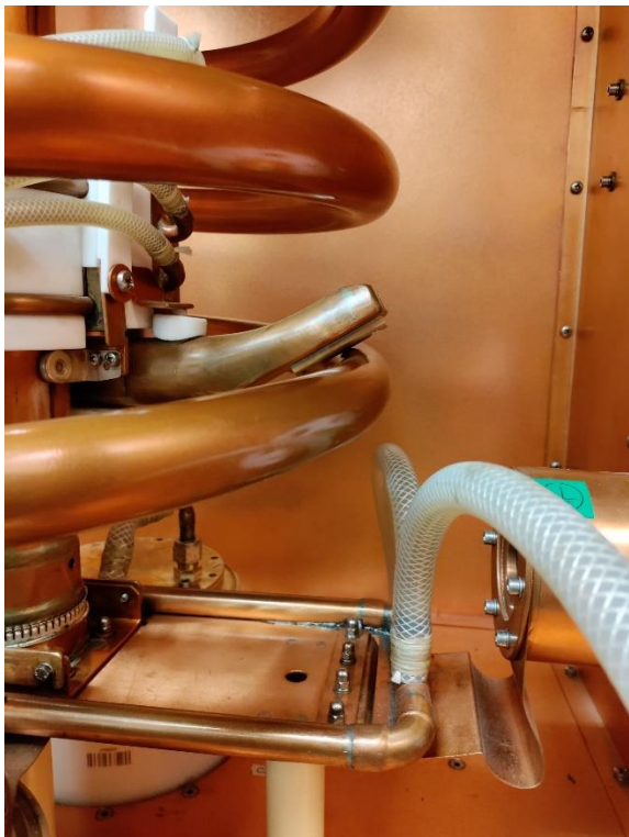
Figure 9. L310 in close-up showing water cooled variable coil tap, and edge of support structure for the assembly which has rounded feature to prevent flashover and is water cooled to prevent RF current burning the edges
