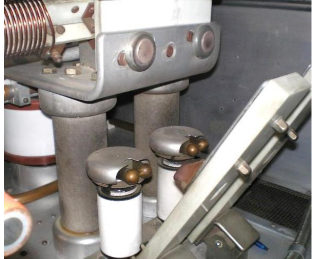
Figure 3. Anti-parasitic capacitor fixings in the MCSL B6124 300 kW final RF amplifier
