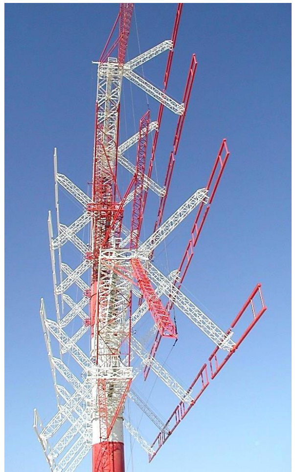
Figure 10. Thomcast rotatable HF antenna. This antenna comprises two 'curtains' of rigidly-supported folded dipoles with a central reflecting screen. The white dipoles are shorter and work at higher frequencies than the darker coloured dipoles. The whole antenna can be rotated to 'point' in the required direction. Photograph courtesy of Pete Bairstow and Babcock Communications
