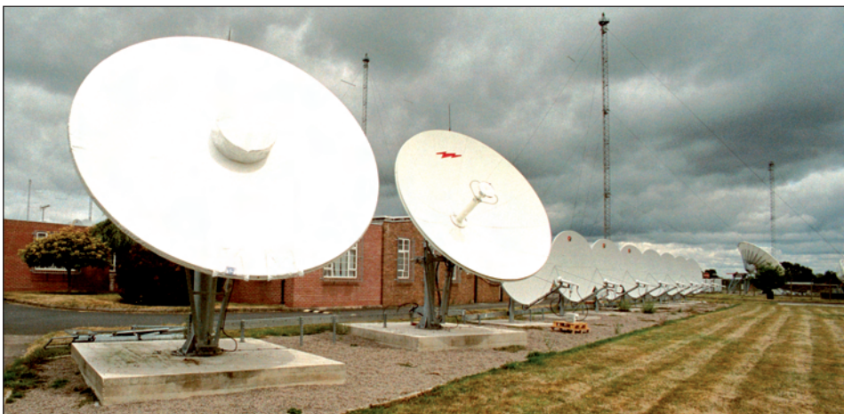
The UK to Kenya Telephone and VOIP satellite link system for Alldean Networks 2010. (Photo by Jeff Cant)
