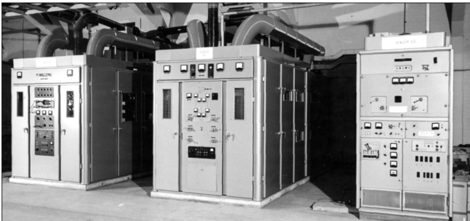
Sender 92, one of the first Marconi 250kW senders, during installation in 1963 (Photo from the Jeff Cant archive)
