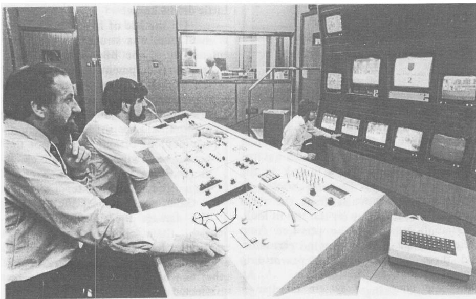
Tom Peckham and Mike Coy (centre) of SCPD seated at the control desk in TV Studio 1, while John Bloomfield, OUPC, adjusts the monitors. John was attached to SCPD for the installation.
