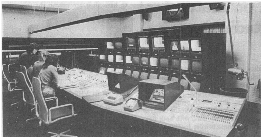
TC2 Production Control Room
