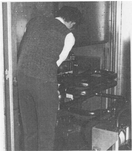
STE Percy Winsor checks the final anode coils inside a transmitter
