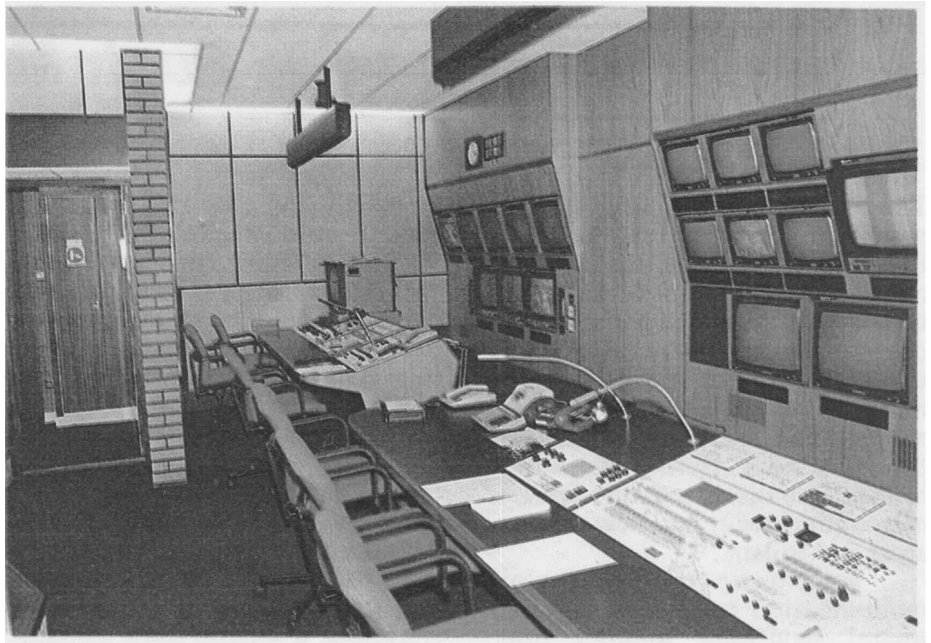
Pebble Mill studio B Production, vision and lighting control areas.
