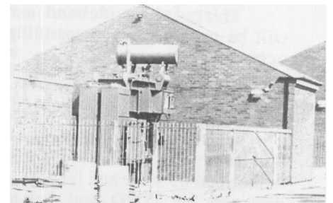
A typical 33 kV/11 kV substation 'ENG INF' Summer 1984 - Page 9
