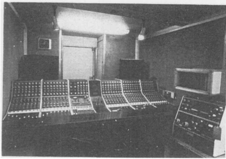
A Calrec 40-channel mixing desk inside a Type B stereo control vehicle
